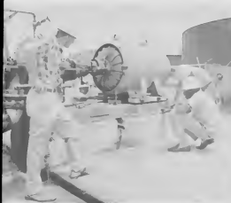
Using a motor-driven centrifugal pump, using clamp-on jigs which allow rapid "hot" measurements without requiring coupling separation. Usando un motor de bombeo centrífuga y usando "clamp-on jigs" cu ta permiti midimento di "calor" rapido sin desconectar e mashinan.
